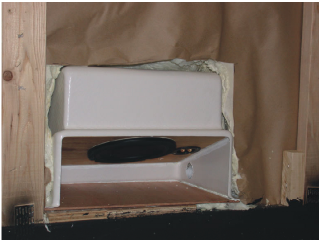
Figure 12. Properly Installed Sub-Woofer
